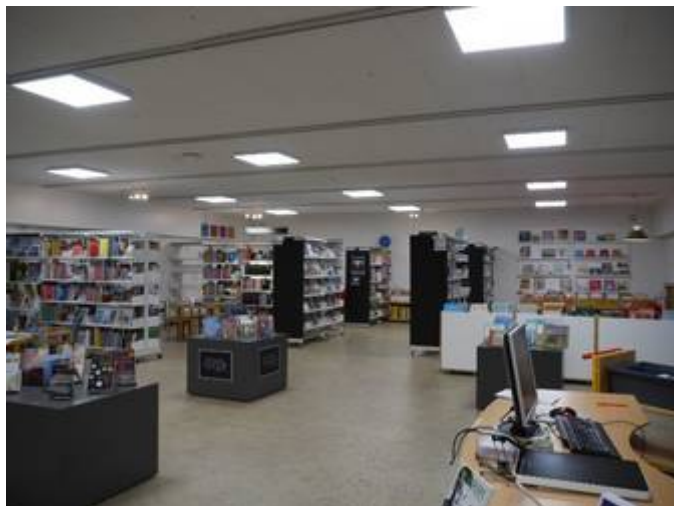
600x600mm LED paneler monteret i kassetter
